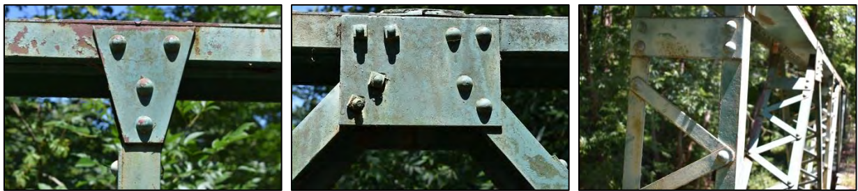
Figure 94: Details of gusset plates, rivets, V-lacing; note bolts in place of rivets at left-hand side of center image
