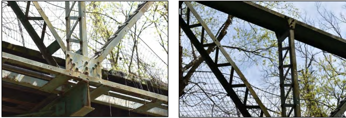
Figure 93: Truss details; note small, regular, empty holes in vertical and diagonal members
