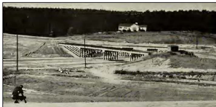
Figure 5: The Beltline under construction in late 1960/early 1961, likely near Western Boulevard ( Roadways Magazine , 1961)
